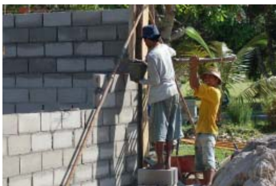
Construction of the new classroom at BCU Photos courtesy of Muhammad Bachrun Bustillo
